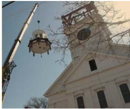
Old South Church Tower Restoration, Newburyport, MA Structural restoration by Structures North, Salem, MA (photo courtesy of Structures North)
